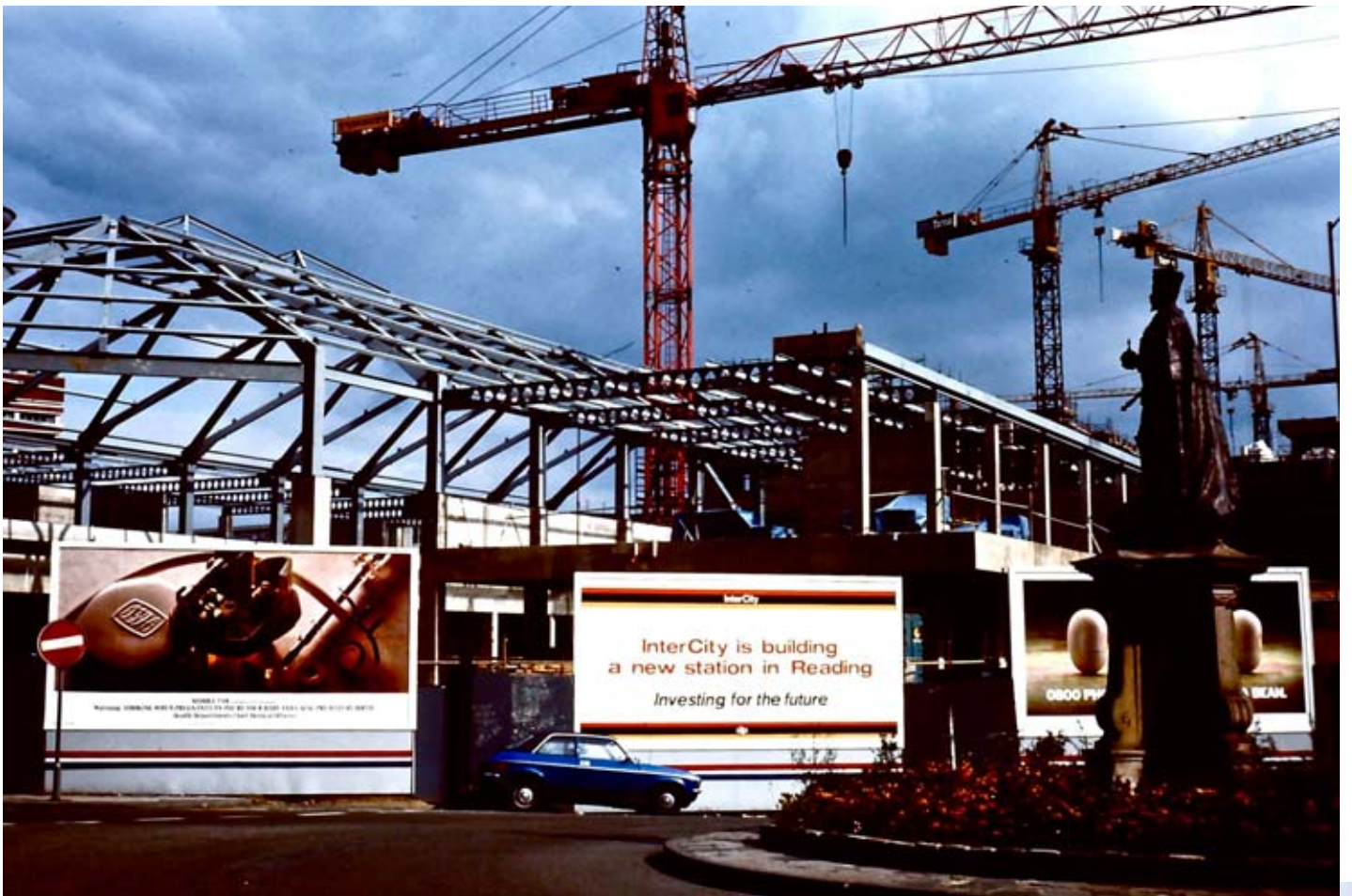
Reading's 1980s re-building, note that InterCity was the sponsor, with Apex Plaza going up to the east.
