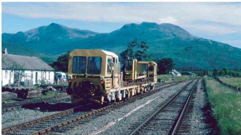
On a day when ASLEF struck and very little moved on the national railway network, General Purpose Track Removal and Maintenance Machine DX98212 takes advantage of a clear road at Strathcarron on the Kyle of Lochalsh branch, 14th July 1995.
